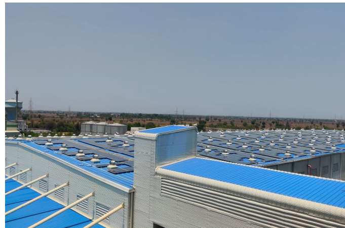
Rooftop Solar at Sayakha Plant
