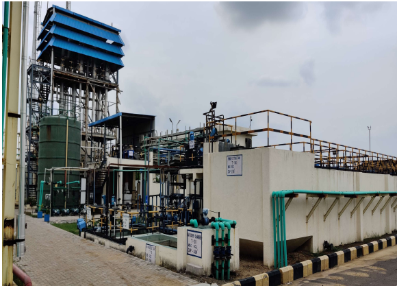
ETP at Sayakha Plant
