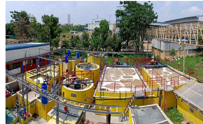
ETP at Hosur Plant
