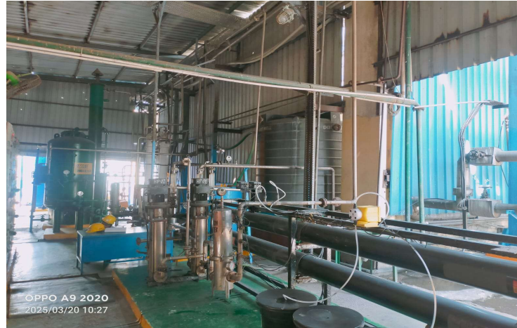
Effluent Treatment at Bawal Plant
