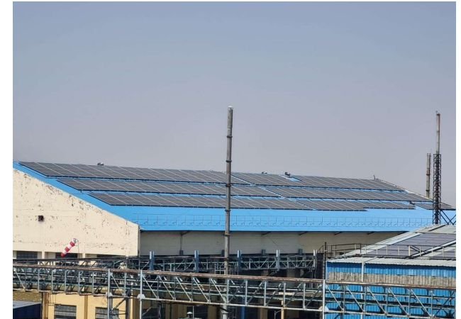
Rooftop Solar at Jainpur Plant
