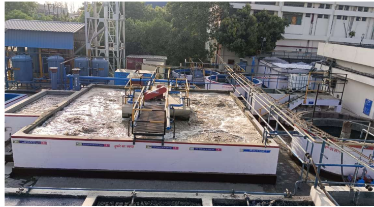
ETP at Jainpur Plant
