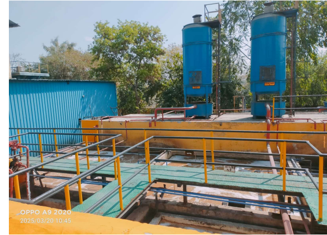
Rainwater Collection inside Bawal Plant Premises
