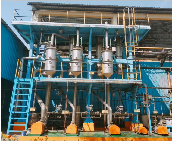
ZLD at Bawal Plant
